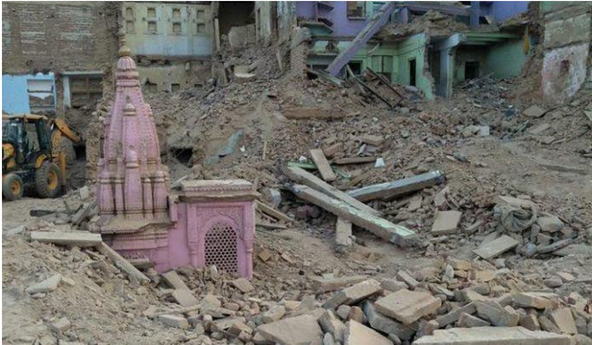
A small temple is revealed as the surrounding caretakers' homes are demolished, photo by Aditi Vatsa.
